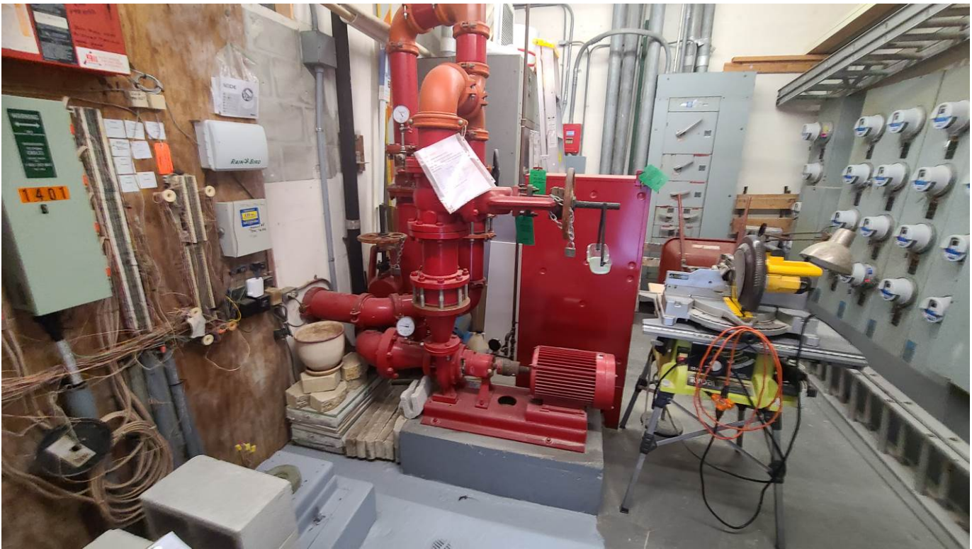
Photograph 19: Building Common Areas – Electrical & Fire Pump Room
