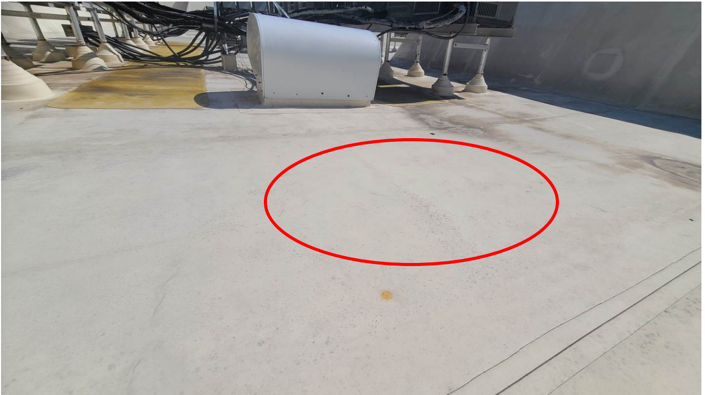
Photograph 9: The Roof – Sample of Roofing Blister.
