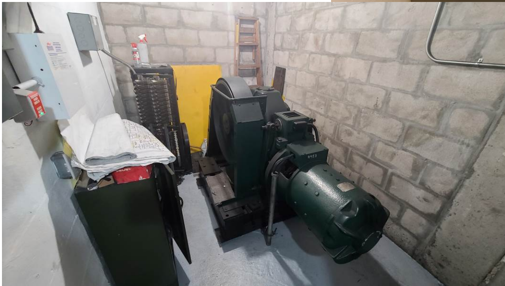
Photograph 18: Building Common Areas – Elevator & Elevator Room
