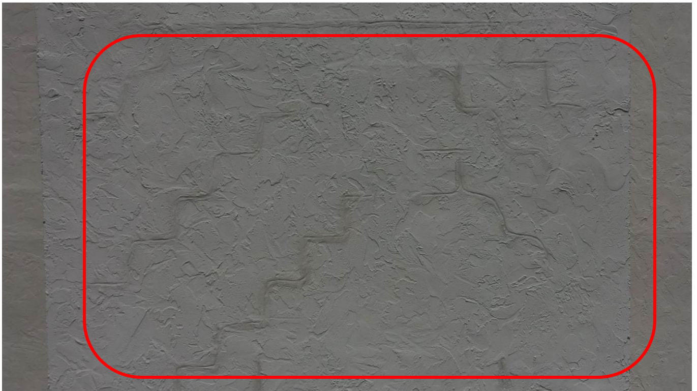
Photograph 6: East Stairwell's Wall at 6 th Level – Sample of Stucco Crack with Signs of Moisture Inside.
