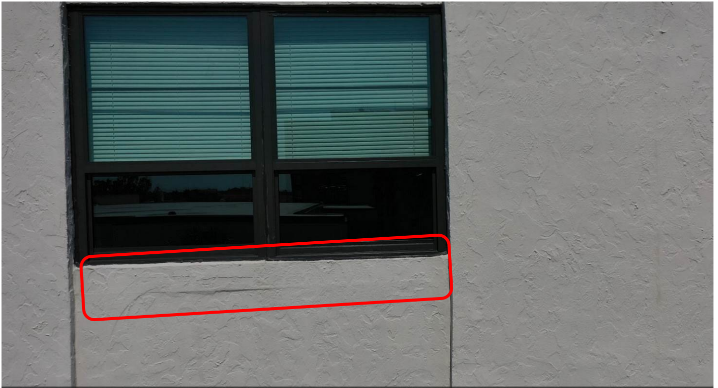
Photograph 5: East Elevation at 4 th Level. 1 st Window from North – Sample of Cracked Window's Sill.
