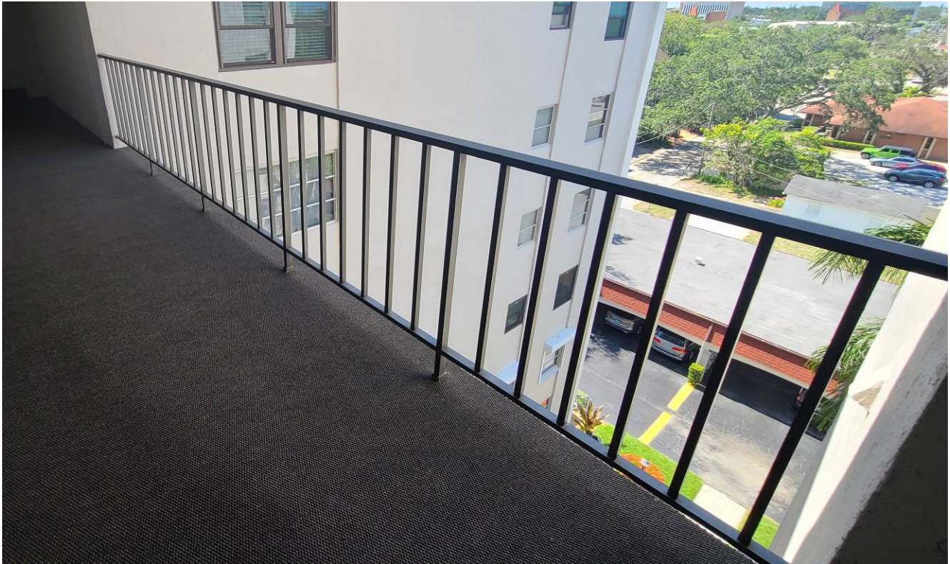
Photograph 16: Typical Walkway Guards. Guards are Mechanically Fastened Members, Core Mounted Posts. Guards Dimensions Do Not Comply with the Applicable Building Code
