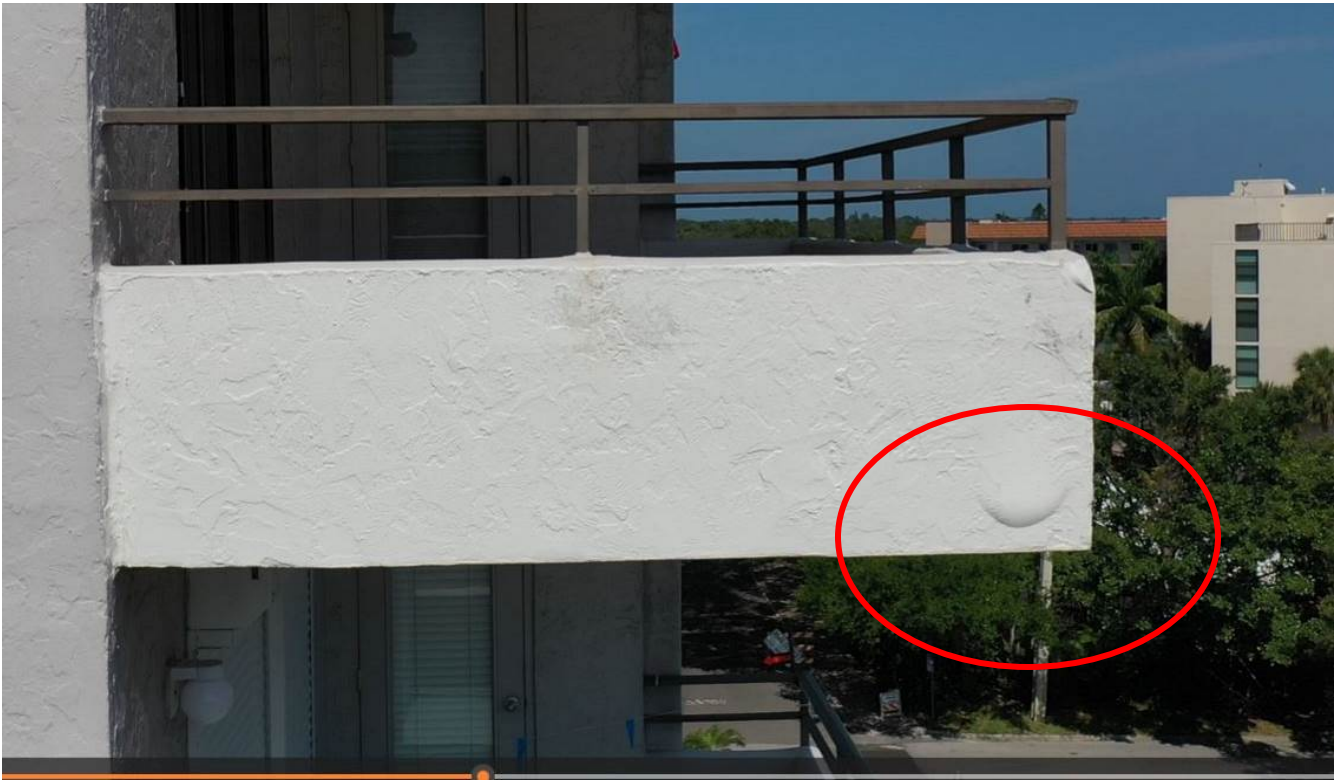
Photograph 7: East Elevation, North Corner Balcony at 6 th Level – Sample of Paint Blister.
