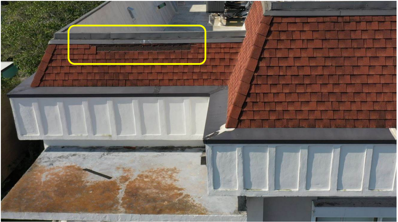
Photograph 11: Mansard Roof (Parapet) – Sample of Missing Shingles on Exterior Face.
